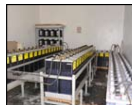
New batteries in place R. Constable
