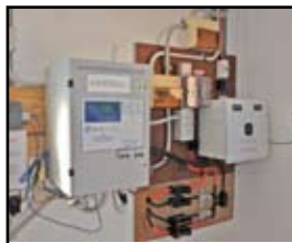
The new inverter in place R. Constable
